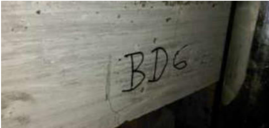
[Fig.5.1: Flexure crack in specimen BD 6 of slab thickness 125 mm]
